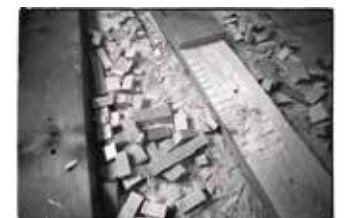
Soon-to-be support beams for the roof structure, with cut-out slots for the sliding windows.
